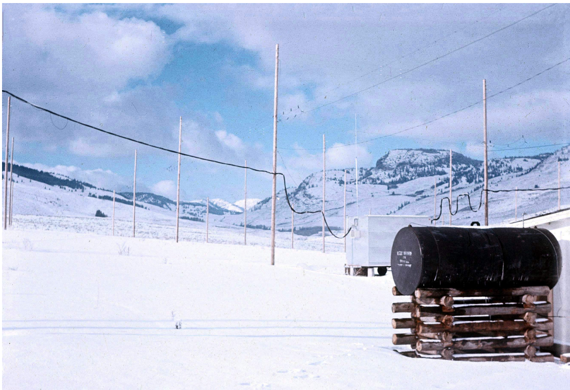
10-MHz array dipoles, trailer and diesel generator fuel tank, January 1966
