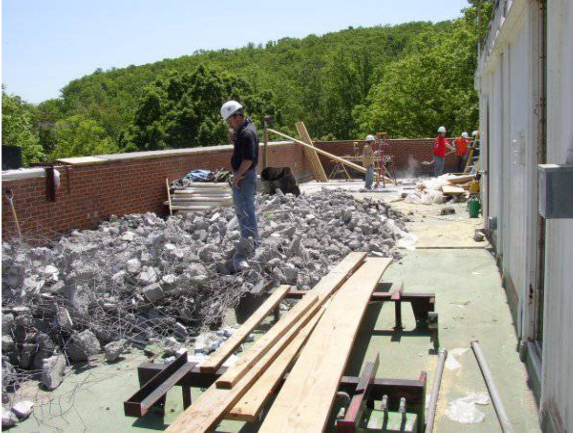
Demolition of the old roof on the East building in May 2004 ... as NRAO staff continued to work below.
